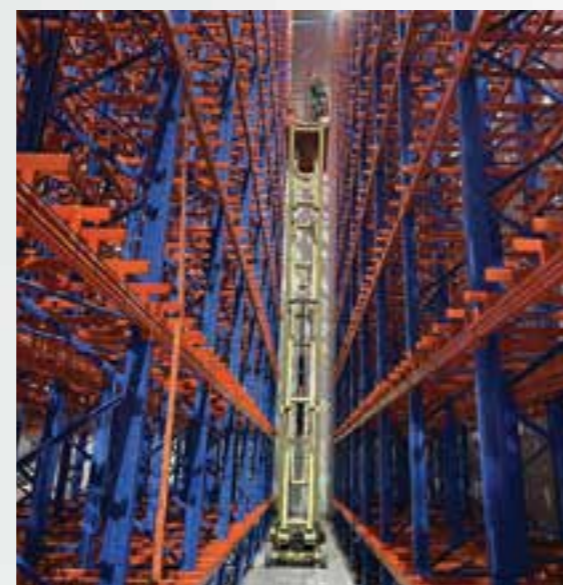
Images of Searefico E&C employees performing operations and installing equipment at the Smart Cold Storage project undertaken by the company.
