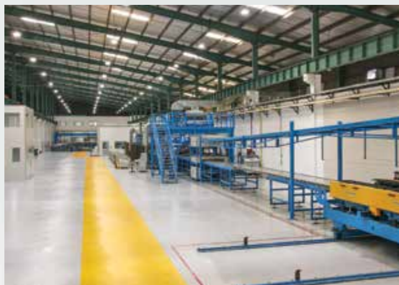
The Panel (PIR) production line, sourced from ITALY, with modern technology is currently operational at the Panel Manufacturing Plant – Greenpan Joint Stock Company.
